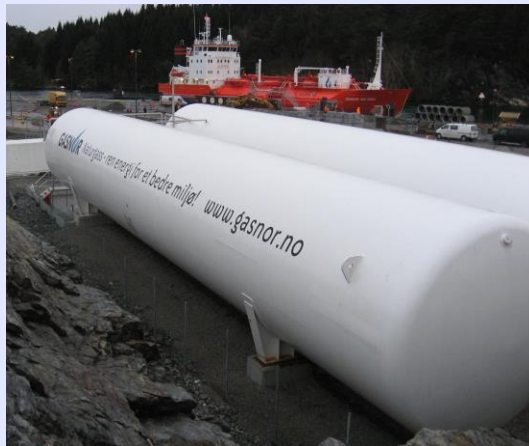
Above-ground, small scale LNG storage for ship fuelling, in Halhjem, Norway
